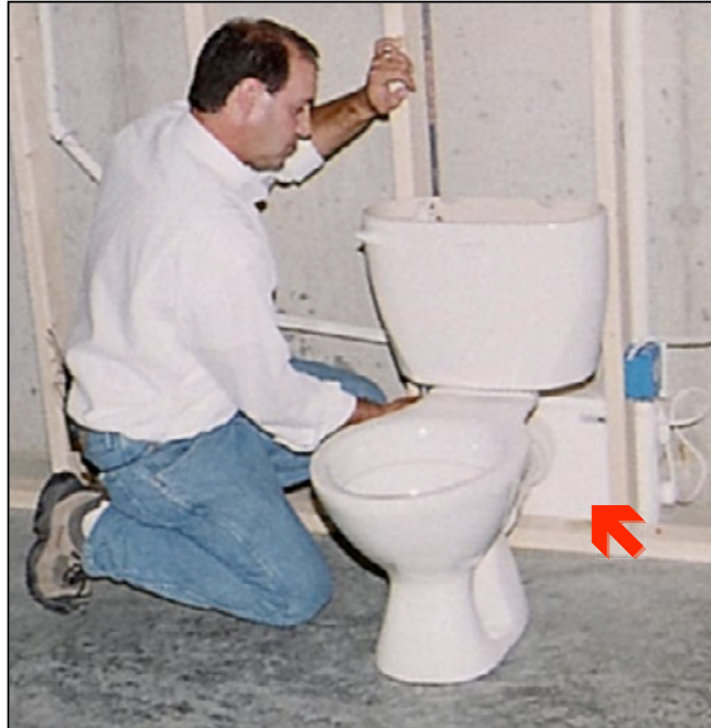
SANIFLO ALLOWS FIXTURE PLACEMENT ANYWHERE, RIGHT ATOP THE FLOOR, WITHOUT BELOW-FLOOR DRAINAGE CONNECTIONS. HERE THE MACERATOR BOX (RED ARROW) WILL EVENTUALLY BE CONCEALED BEHIND THE WALL.
