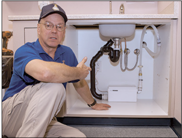
CONTRACTOR JOHN MORRIS, WITH ONE OF THE SANIFLO SANISHOWER GRAY WATER PUMPS. USING CONVENTIONAL PLUMBING TECHNIQUES ON THIS PROJECT WOULD HAVE ENTAILED "A HUGE AMOUNT OF WORK," HE SAYS. "IT WOULD HAVE TAKEN US AN ADDITIONAL THREE MONTHS."
